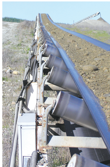
A 30-inch wide electric-powered conveyor with enclosed self-lubricating rollers transfers material to processing at the Shine Pit.
